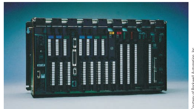
FIGURE 53-8B I/O rack with input and output modules.
